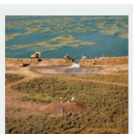
Work to cut a hole in the sea wall in Tollesbury, Essex, in the 1990s as part of a saltmarsh restoration scheme (Picture: Natural England)
