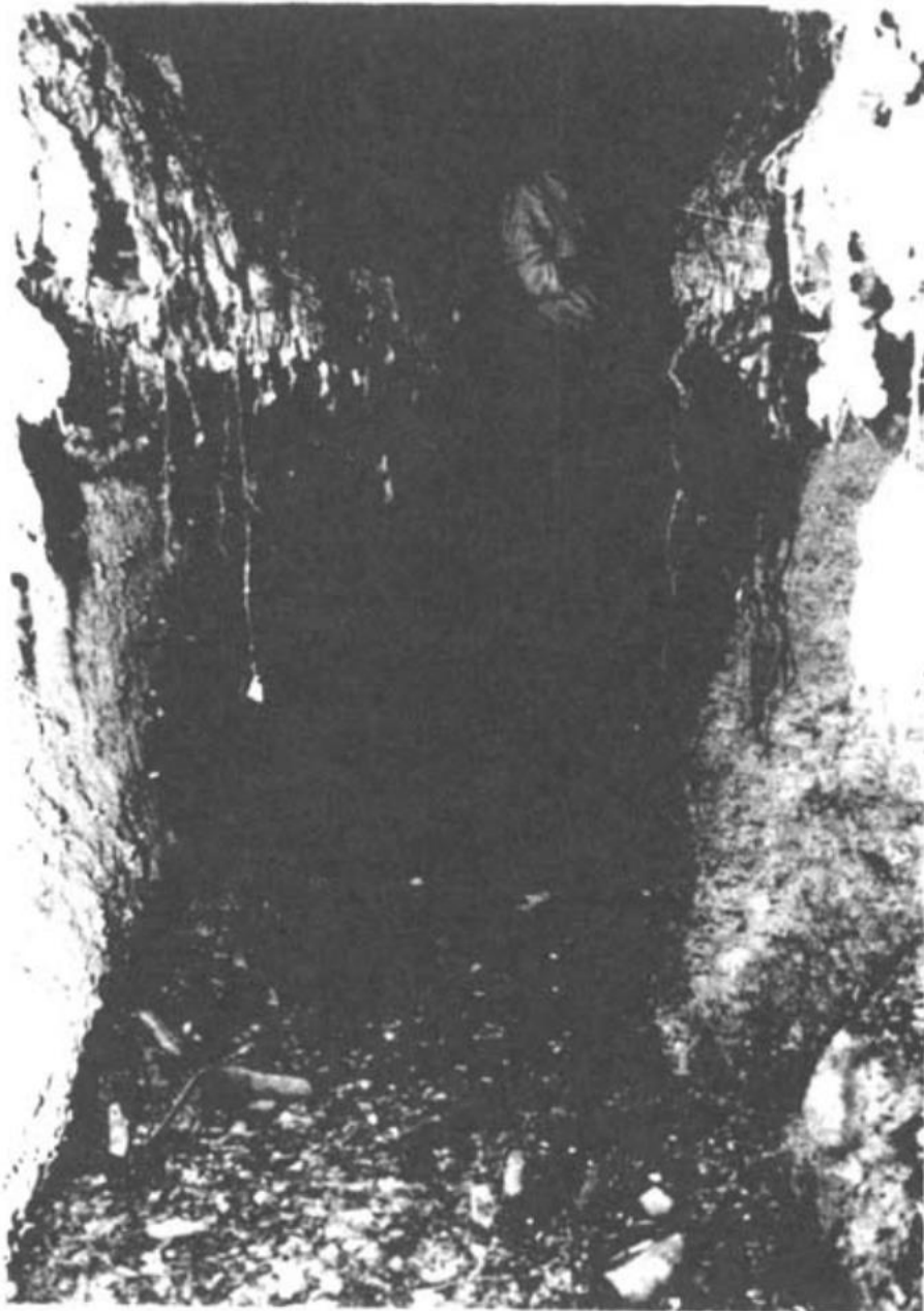
Appendix 2: Severely eroded drainage ditch in the Tanllwyth catchment. Taken from Newson (1980b).
